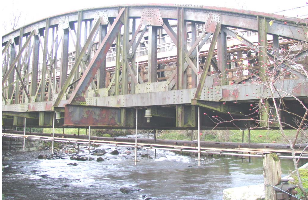
Scaffolding and boards under one of the river bridges during previous inspections and repairs.
