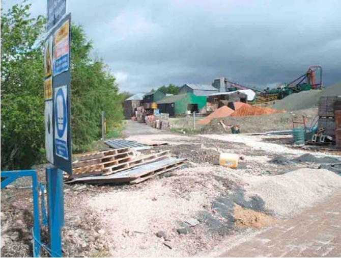
Trackbed east of the block yard, past the carbon works, towards Penrith. Untidy, perhaps, but not obstructed.
