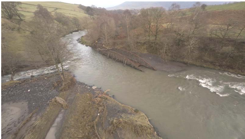
Bridge No. 71 at Brundholme Woods swept off its abutments but recoverable Photograph Copyright © Terry Abraham
