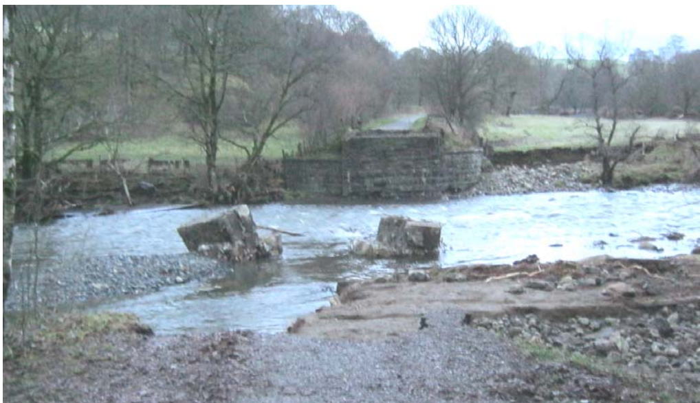
The gap left by the destruction of bridge No. 66. Photograph © Cedric Martindale.
