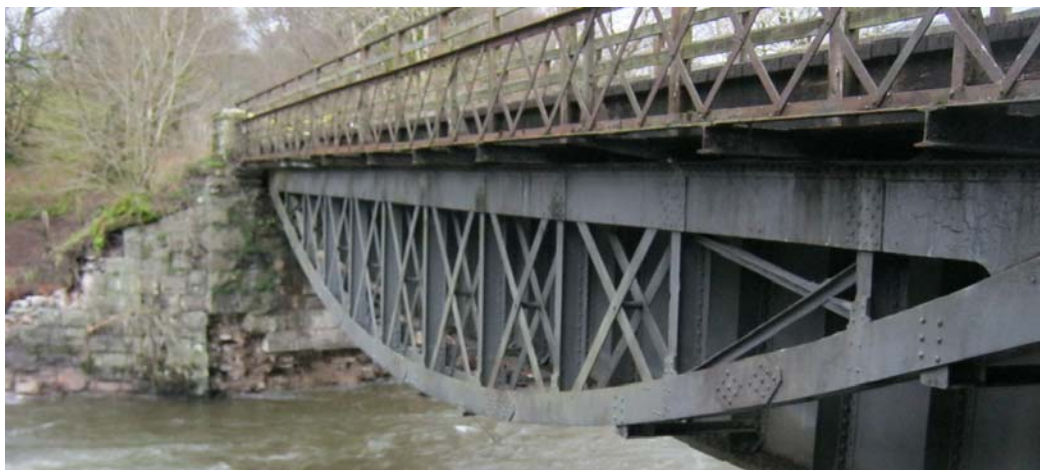
Damage to the western abutment of bridge No. 73 at Rawsome. Photograph © Cedric Martindale
